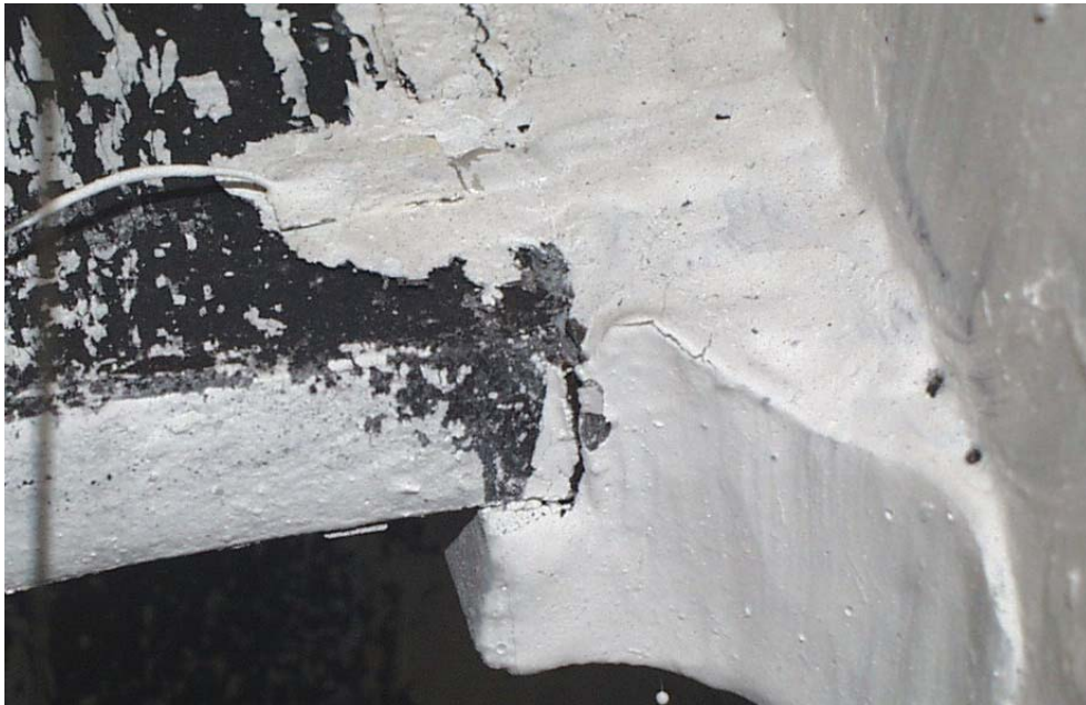
(b) Fracture initiation at west edge of top flange (0.13-1P)
