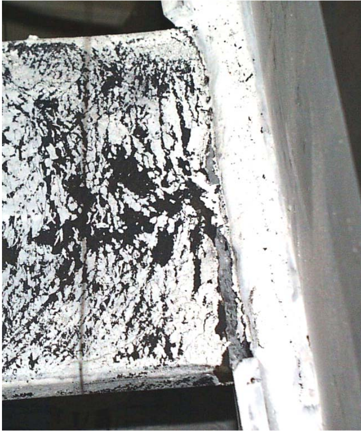
(a) Fracture in link top flange (0.03-2P)
