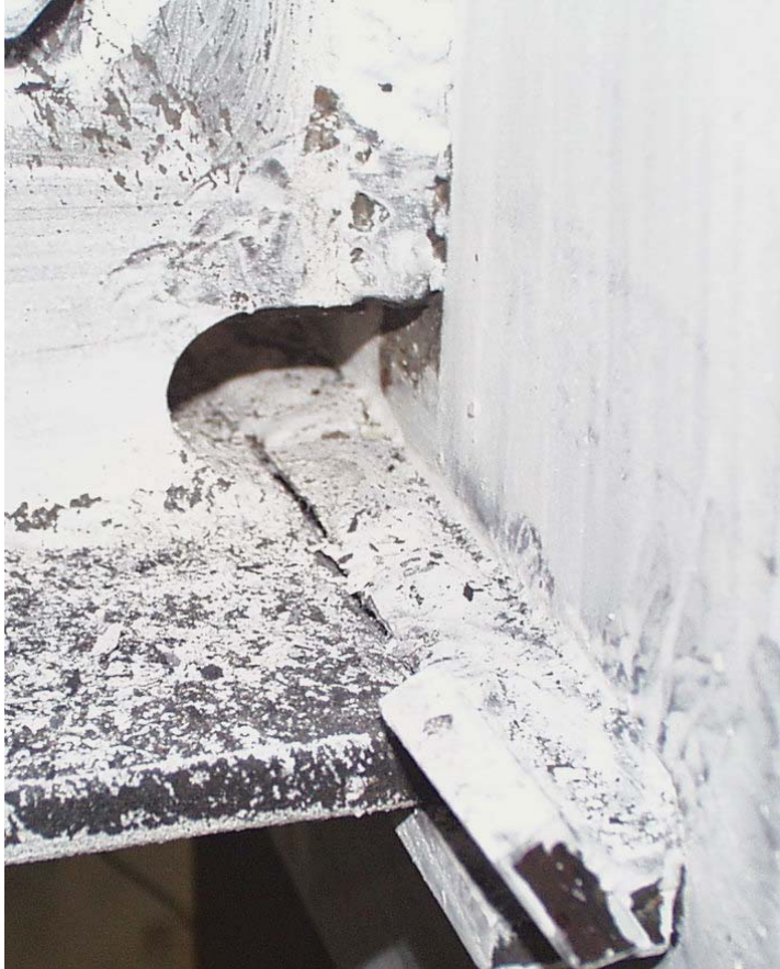
(a) Fracture in link bottom flange (0.02-2N)
