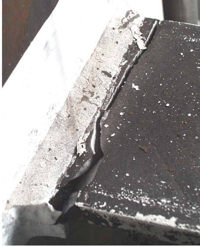
(b) Link top flange separated from column flange (0.04-1P)
