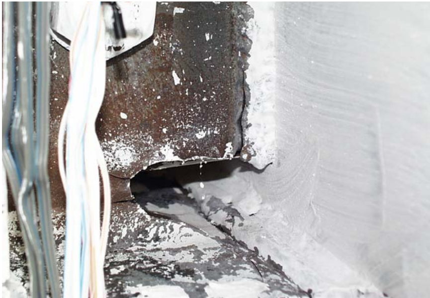
(b) Fracture at bottom edge of link web (0.07-1N)
