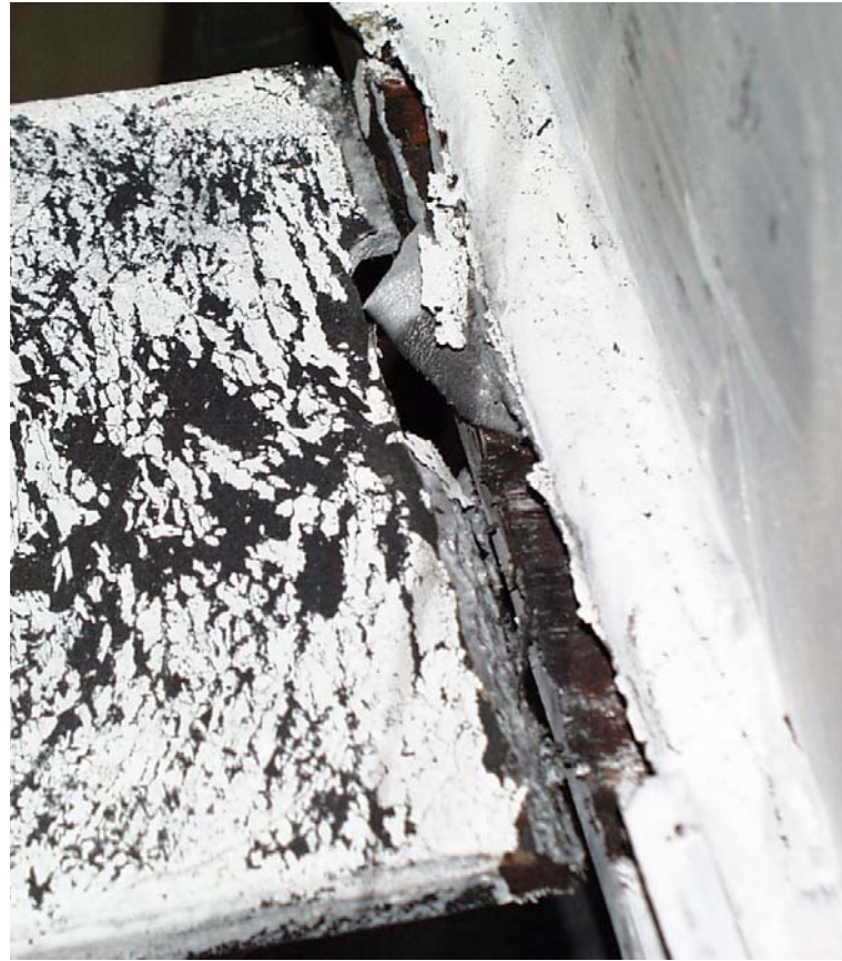
(b) Link top flange separated from column flange (0.04-1P)
