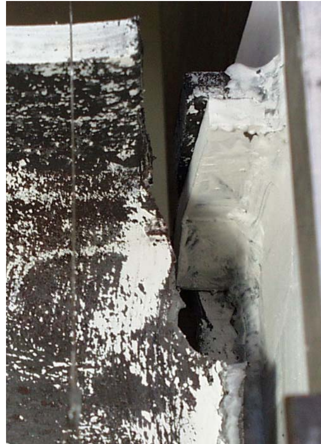
(d) Side view of link top flange separated from column flange (after test)
