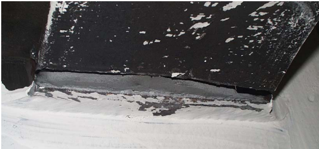
(d) Link bottom flange separated from column flange (after test)
