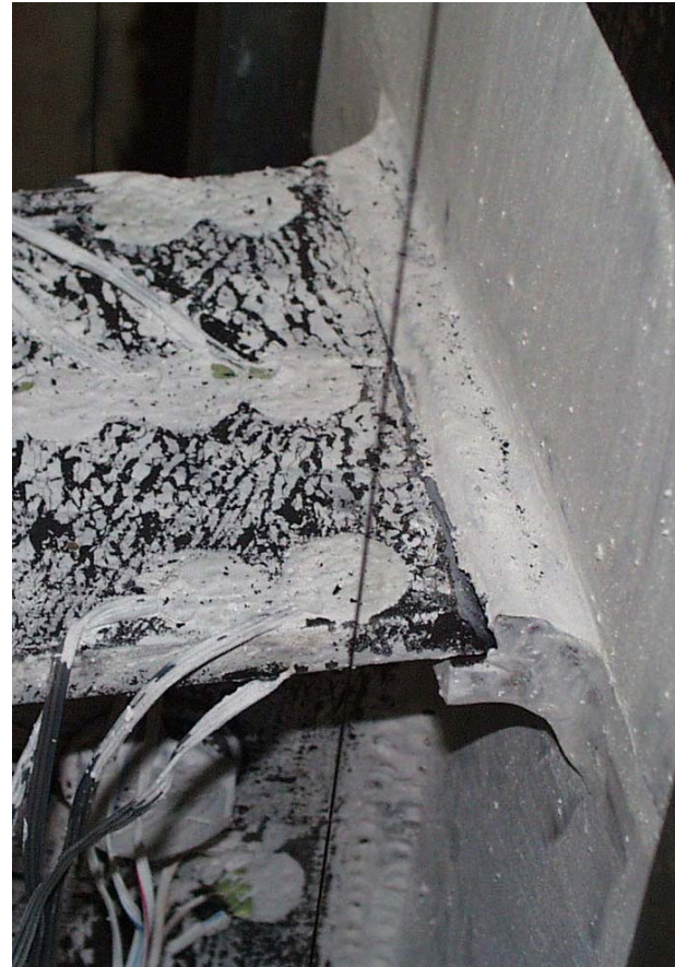
(b) Fracture in link top flange (0.04-1P)
