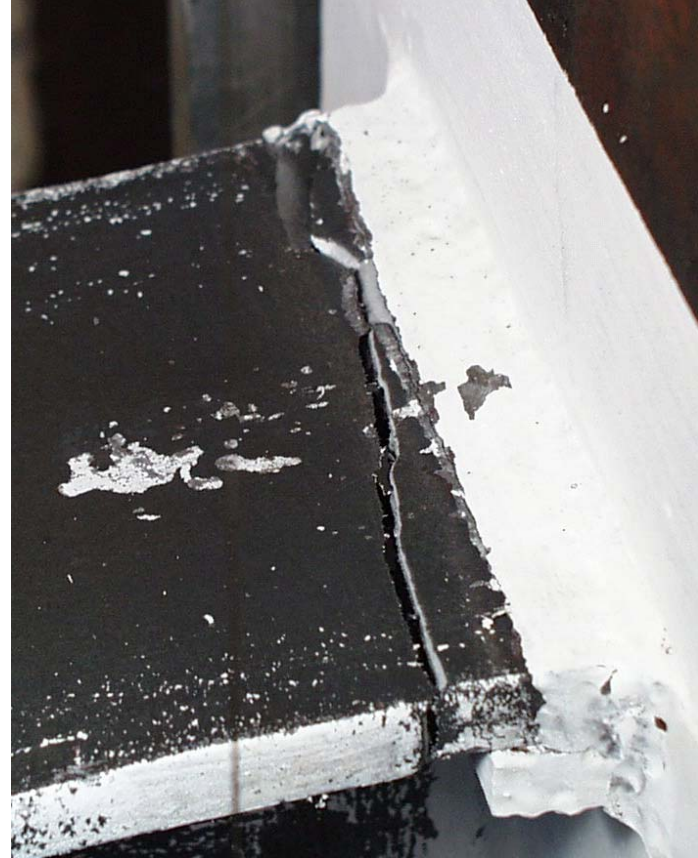
(b) Link top flange separated from column flange (0.05-1P)
