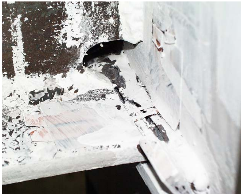
(a) Fracture in link bottom flange weld (0.05-2N)
